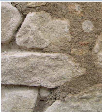
Modern lime mortar pointing, Scottish Lime Centre, Charlestown, Fife. The use of lime allows the wall to 'breathe'. Traditionally, most rubble walls had lime slastered, or buttered, over the joint to achieve a fairly smooth finish that would erode with time. Where pointing does not alter the character of a listed building it would not normally require consent.
